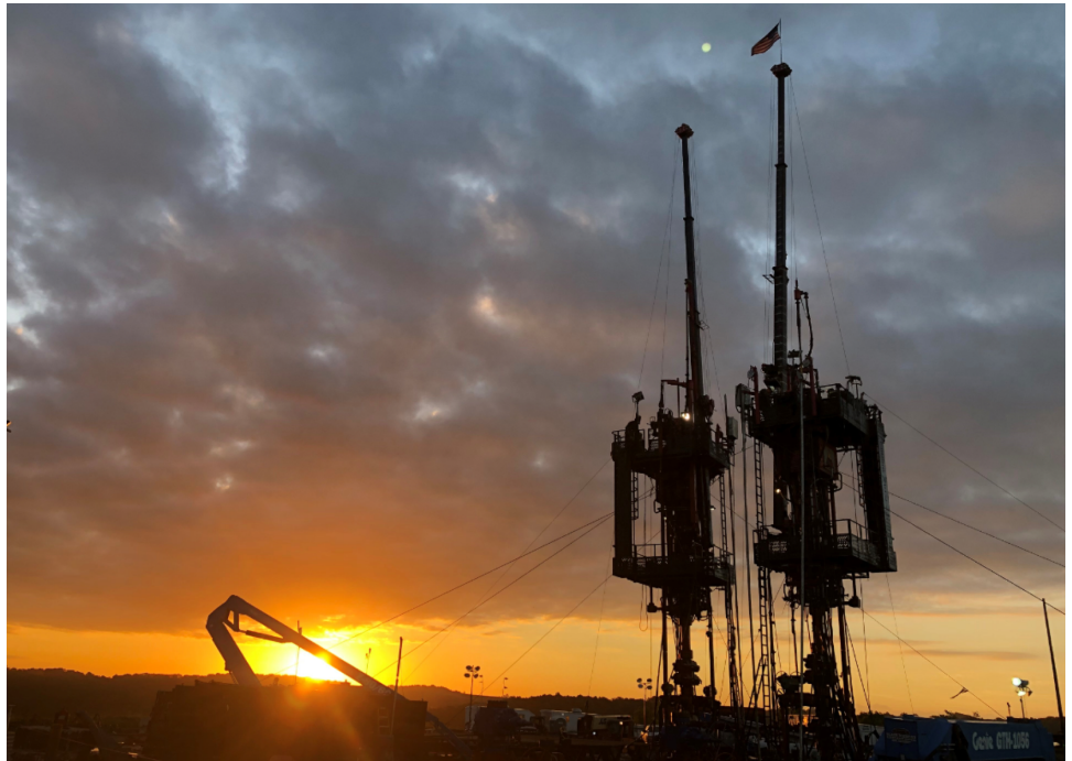
Figure 1: Hydraulic Completion Units (HCUs)
